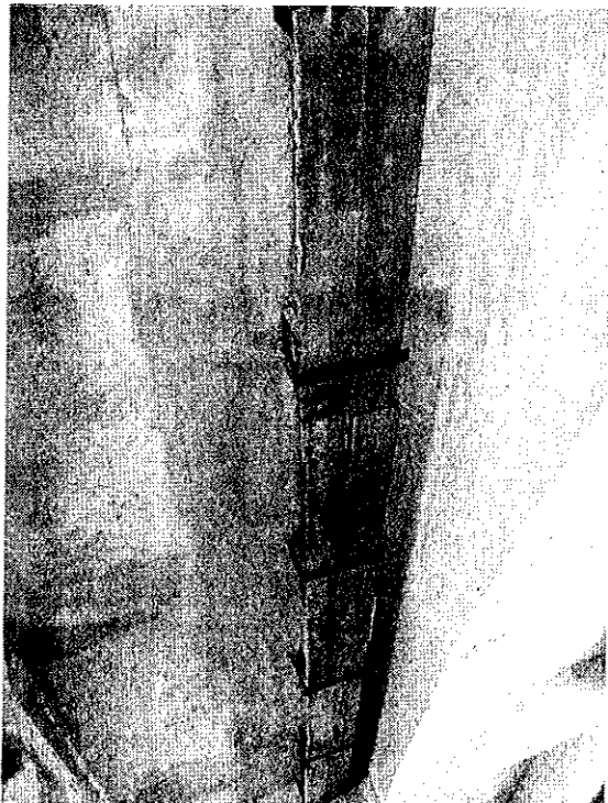
Photo 18 (IMG-1067) – Utility along underside of north span. Note extensive patching in area of duct.
