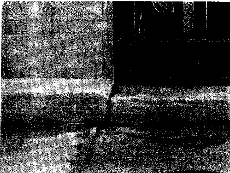
Photo 8 (IMG-1047) – View of north east approach sidewalk. Note settlement.
